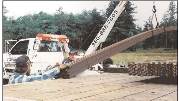
Rod, from Royal Towing, lifting a bundle of 12 lb. rail off of a flat bed truck. Rail is 30 feet long and there were 32 rails per bundle.
