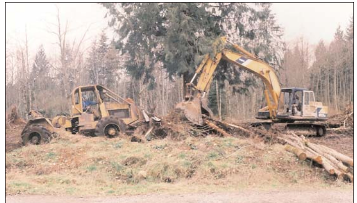
Terry, my logger, on the excavator, and Roy, on the skidder, clearing future site of the depot.
